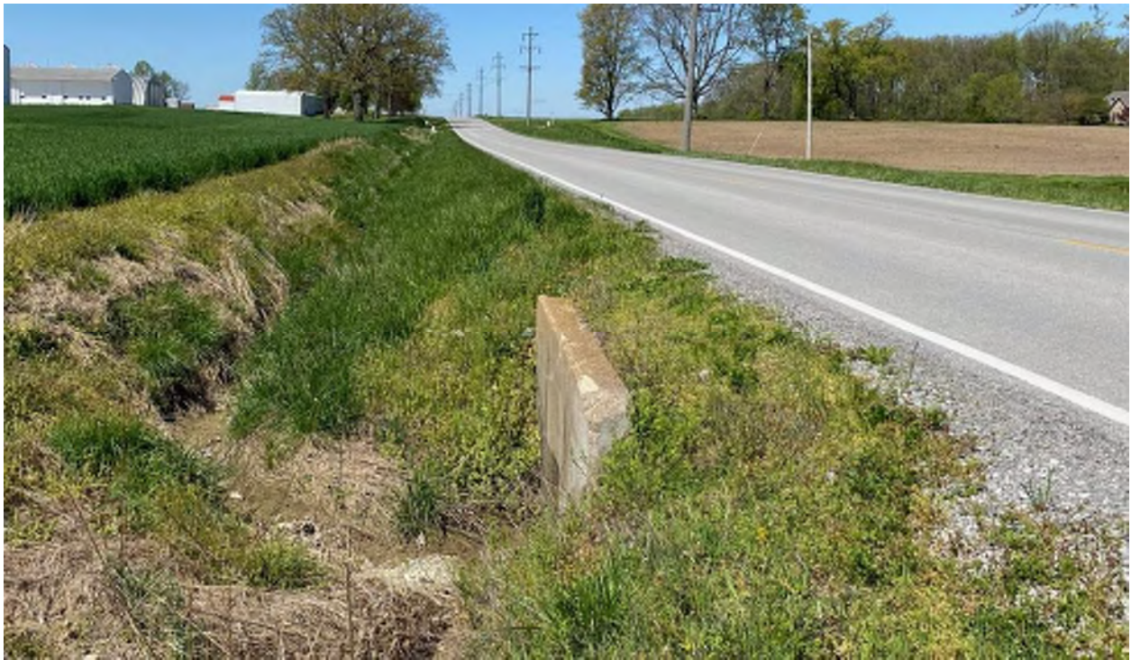
PHOTO 5: CULVERT HEADWALL CRASH LOCATION (MILE 4.65)
