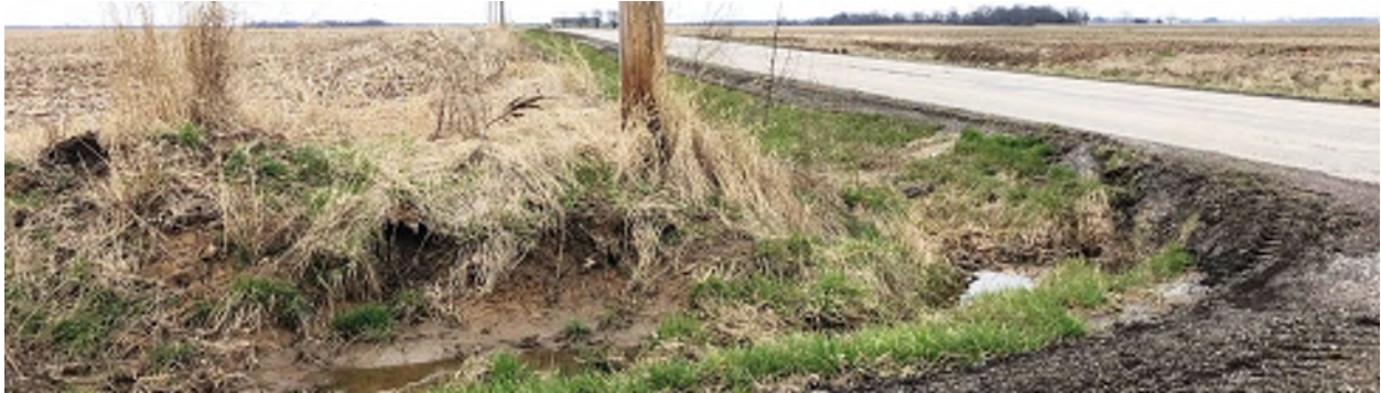
PHOTO 3: DROP OFF AND REPAIR WEST OF RAILROAD CROSSING (MILE 1.95)
