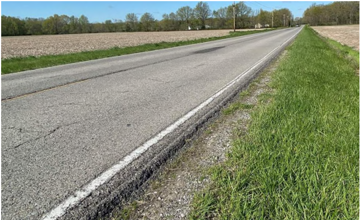
PHOTO 1: SHOULDER DROP-OFF EAST OF FAIRDRIVE LANE (MILE 4.60)
