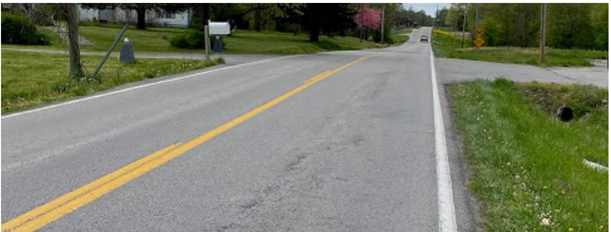
PHOTO8: NO SHOULDER ON WB GREENS MARKET ROAD (MILE 5.70)
