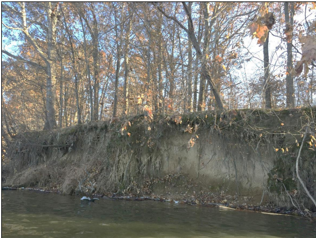
Figure 2.47 - Carbondale Reservoir Severe Erosion
