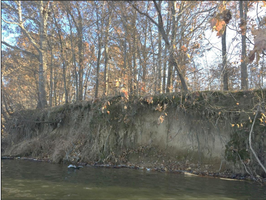
Figure 7.18- Carbondale Reservoir Severe Erosion
