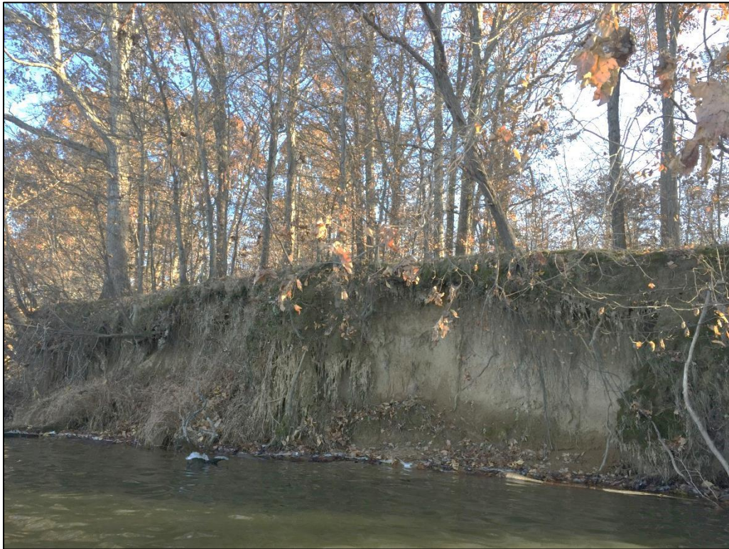
Figure 7.18- Carbondale Reservoir Severe Erosion
