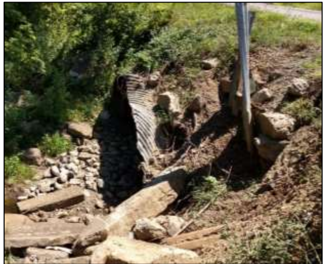
Figure 50 – Deteriorating Culvert in Lake Creek Watershed
