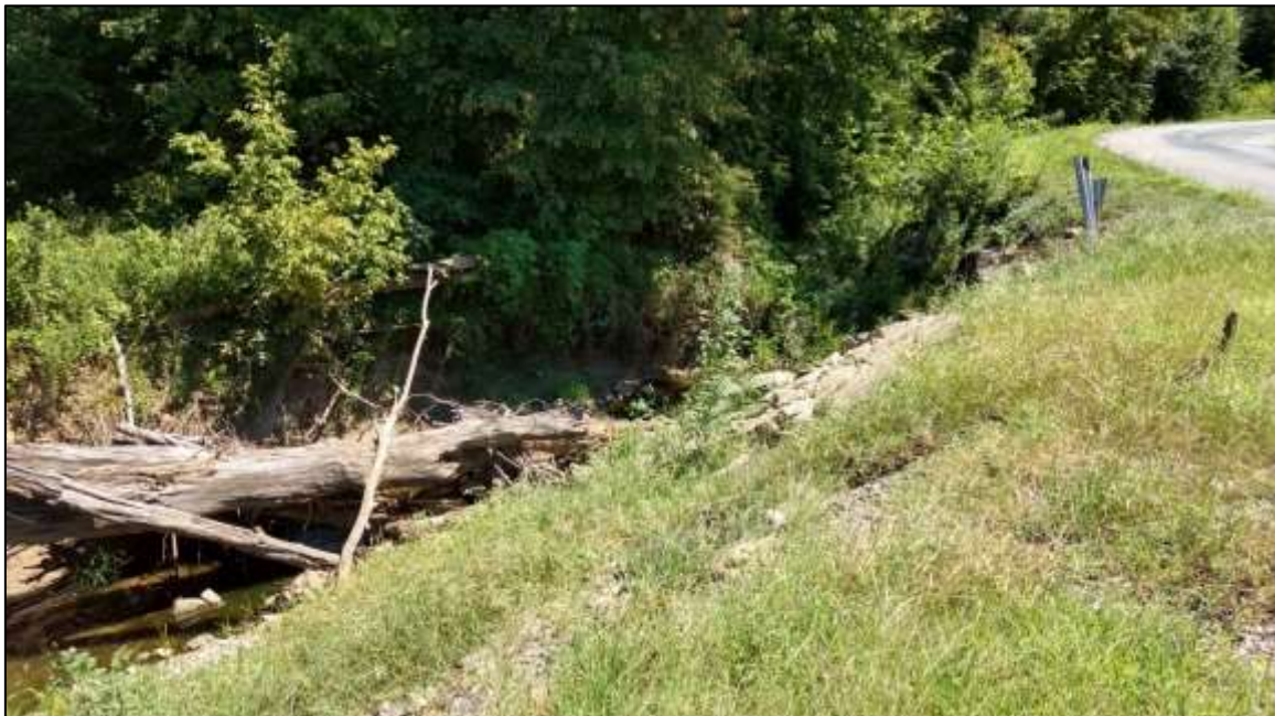
Figure 30- Natural Debris Blockage (Whiteash Branch)
